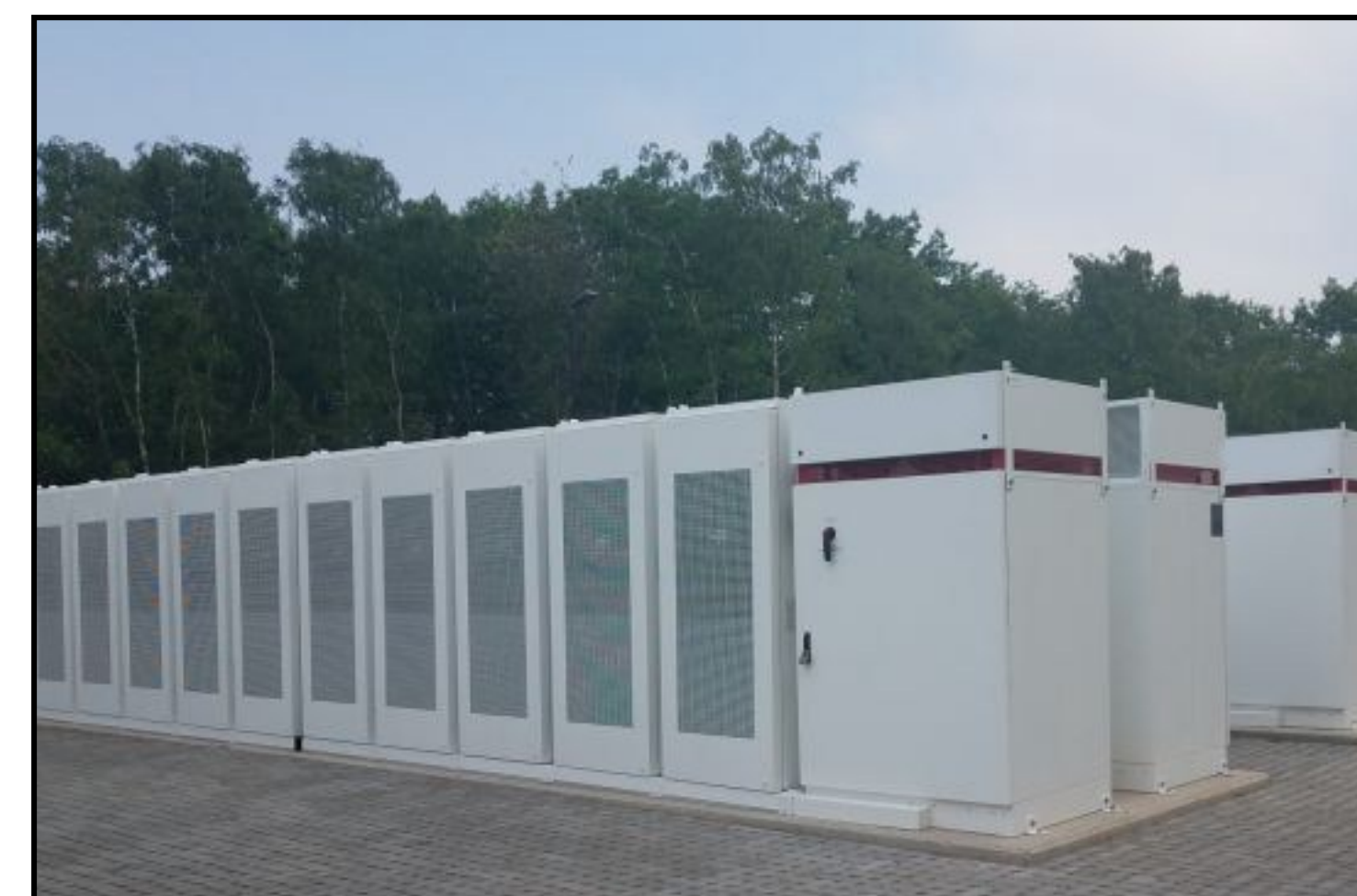
Example Battery Storage Units
