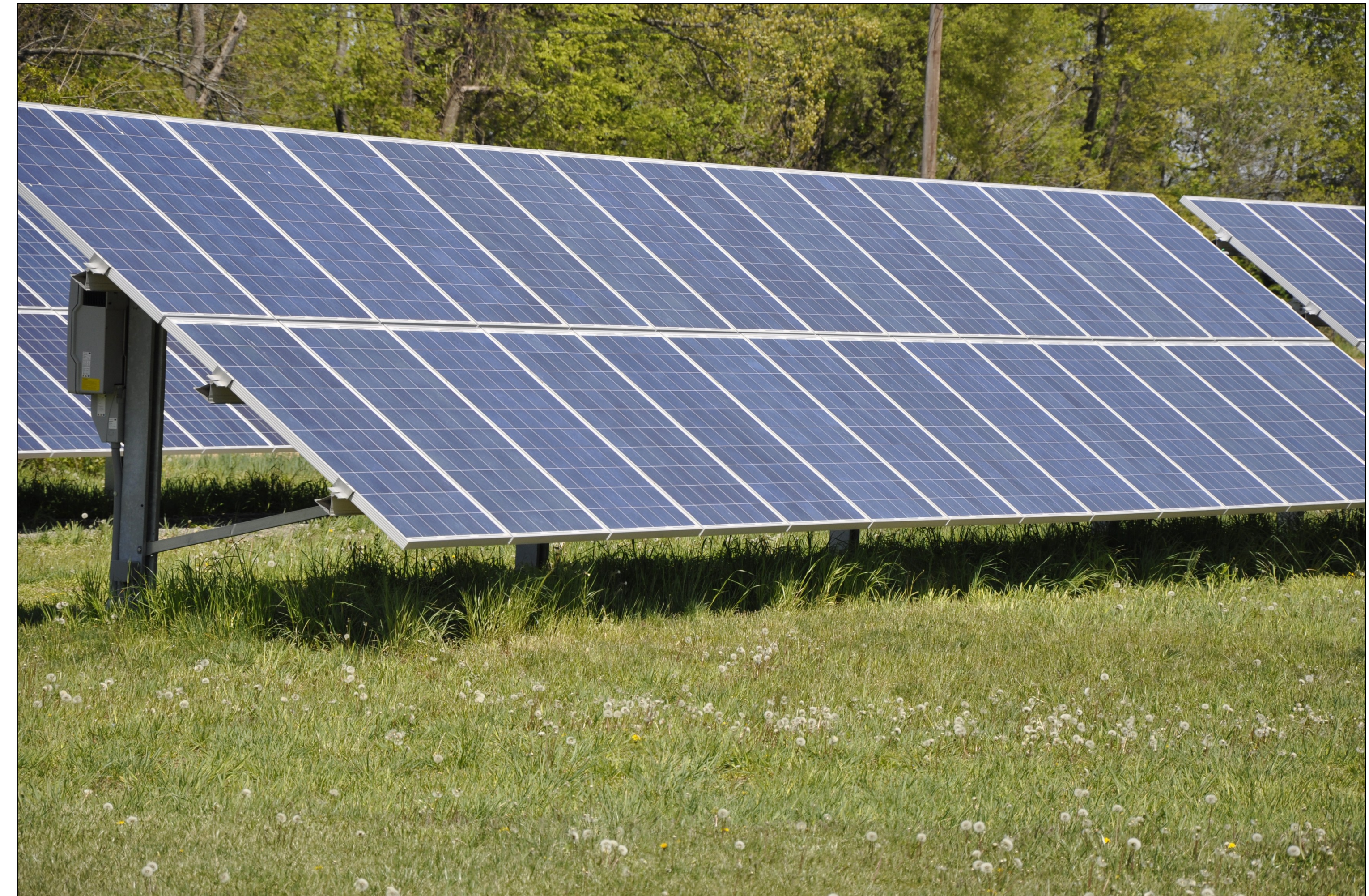
Ground-mounted solar panels
